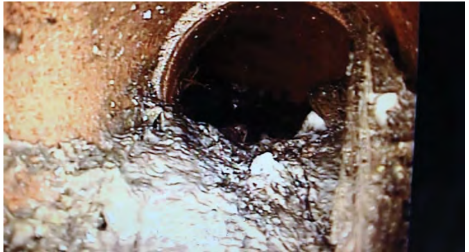
above: grease buildup in lateral
