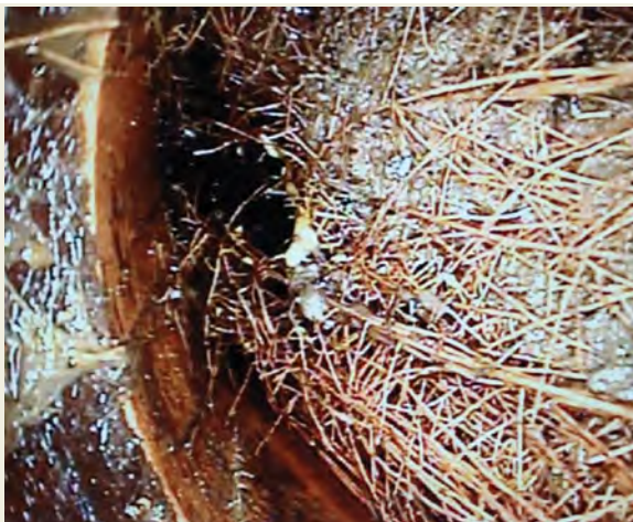
at right: root intrusion in homeowner laterals
